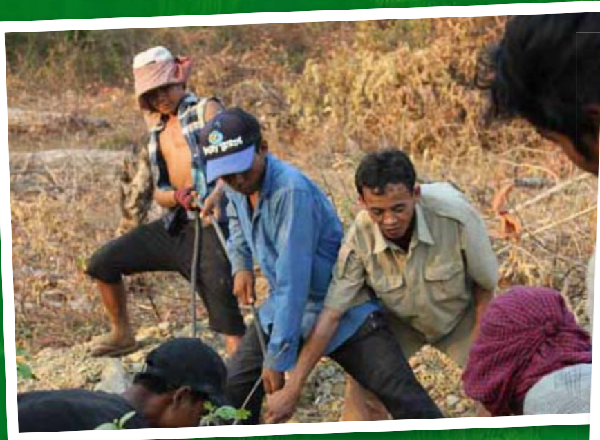
This is where we build the materials for toilets with Oxfam's support. We are building the last toilets now.
